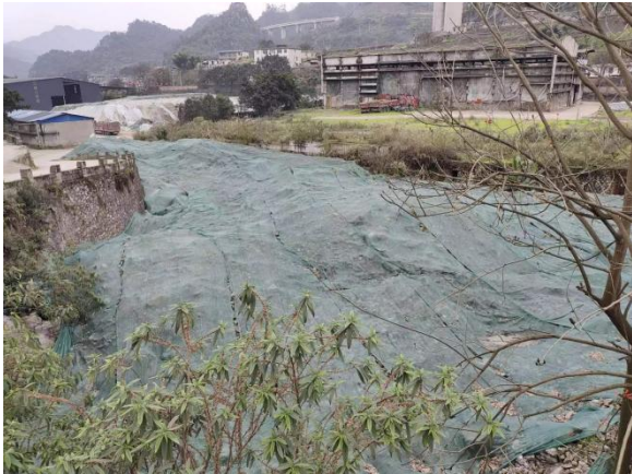
备品备件库、危废间、配电房、淋溶水收集池区域建渣
